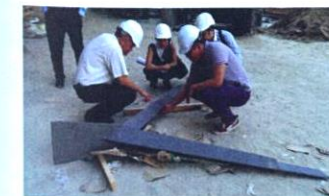
The forked strut of the entrance glass wall, though appearing lightweight, is of considerable dimension adequate in providing lateral stability
